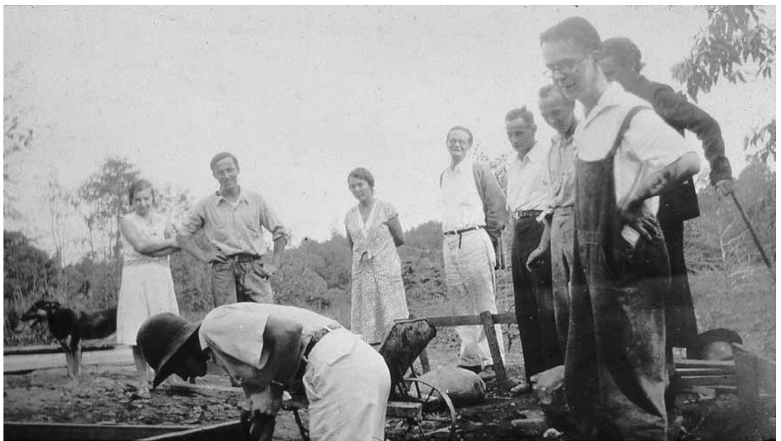
Laying the cornerstone to the Heckel house in 1934, Fred Heckel standing in front with overalls; house designed and built by Fritz Westhoff (third from right standing)
